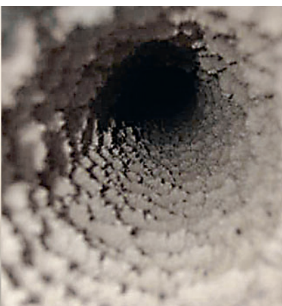
Tuyau flexible encrassé
